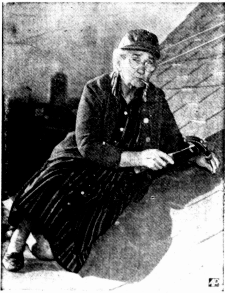
NEVER TOO OLD —Roofing is all in the day's work for Mrs. Verdle Scott of Midland, Tex. The 75-year-old widow does roof repairs, electrical work and is a licensed plumber.
