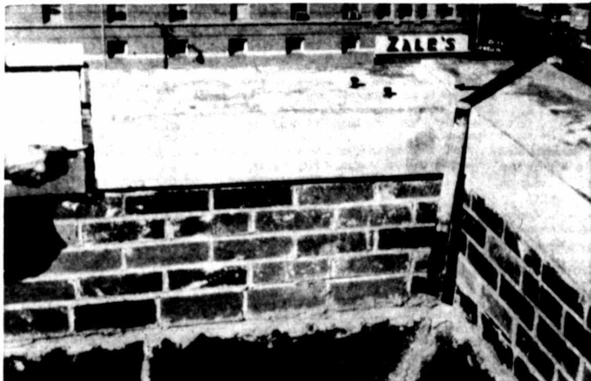
What Cracked The Roof Ledge?
