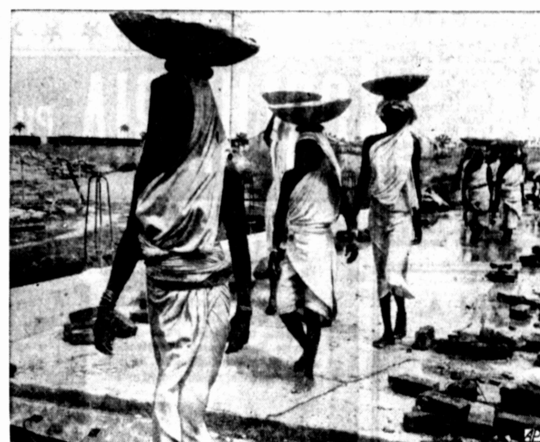
CONCRETE CONVEYORS — Women workers carry pans of concrete on their heads for the construction of a bridge at Durgapur, an eastern Indian area being industrialized.
