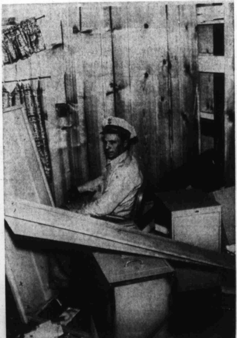
FIRE CAPT. A. D. MEADOR SURVEYS DAMAGE Blast wrecked office building at 1606 Donley today
