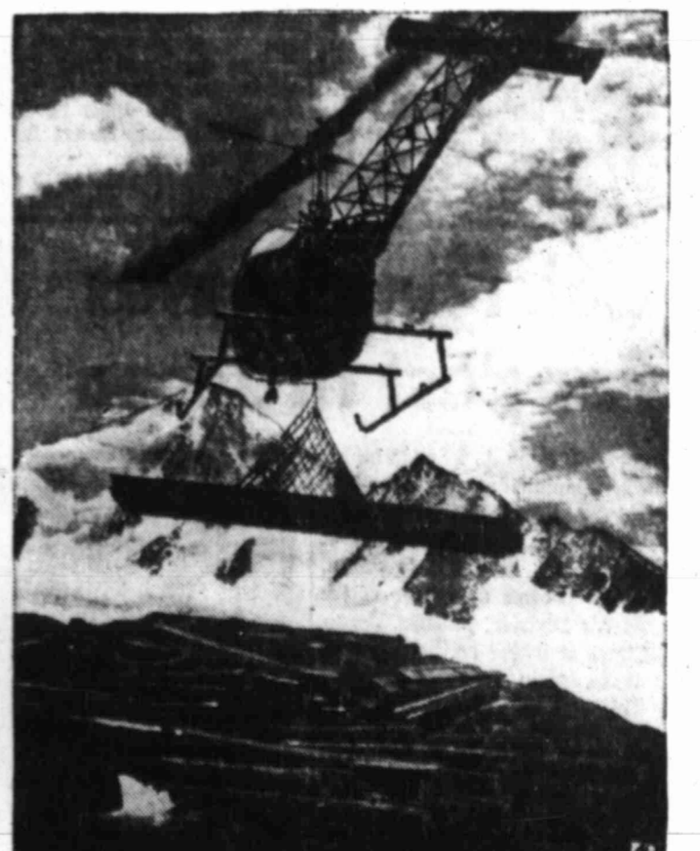
THE ALPINE LIFT — Building materials really come high in the French Alps as a helicopter totes lumber for shelter on 12,500-foot-high peak in the Charbonnet Aiguille.
