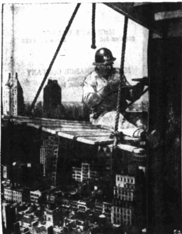
LOFTY OUTLOOK — Dan Weugrenuk, 63, is a man accustomed to high altitudes and precarious perches as he works on 30-story level of Canada House going up in mid-Manhattan.
