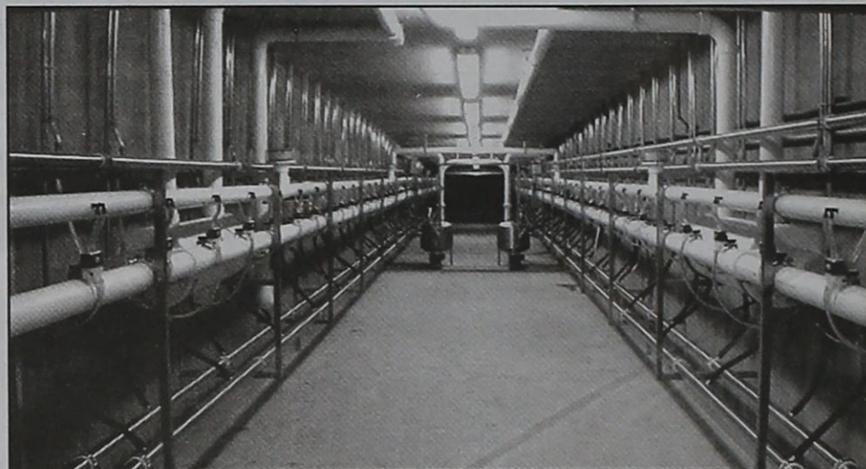
3-H PROGRESS DAIRY USES an underground milk collection system. The system is below ground level for increased cleanliness.
