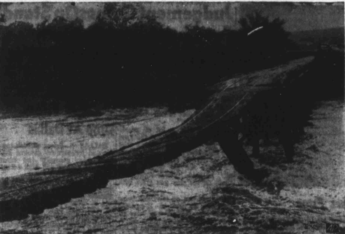
Trestle Almost Gone
