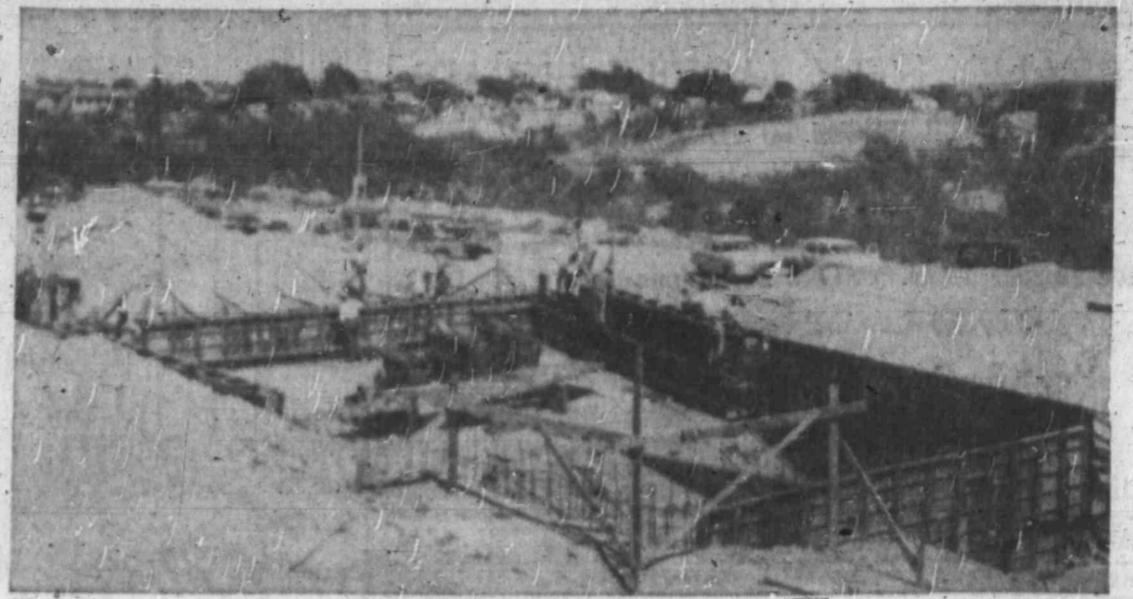
NEW SWIMMING POOL TAKING SHAPE Workmen set concrete walls in Negro park.
