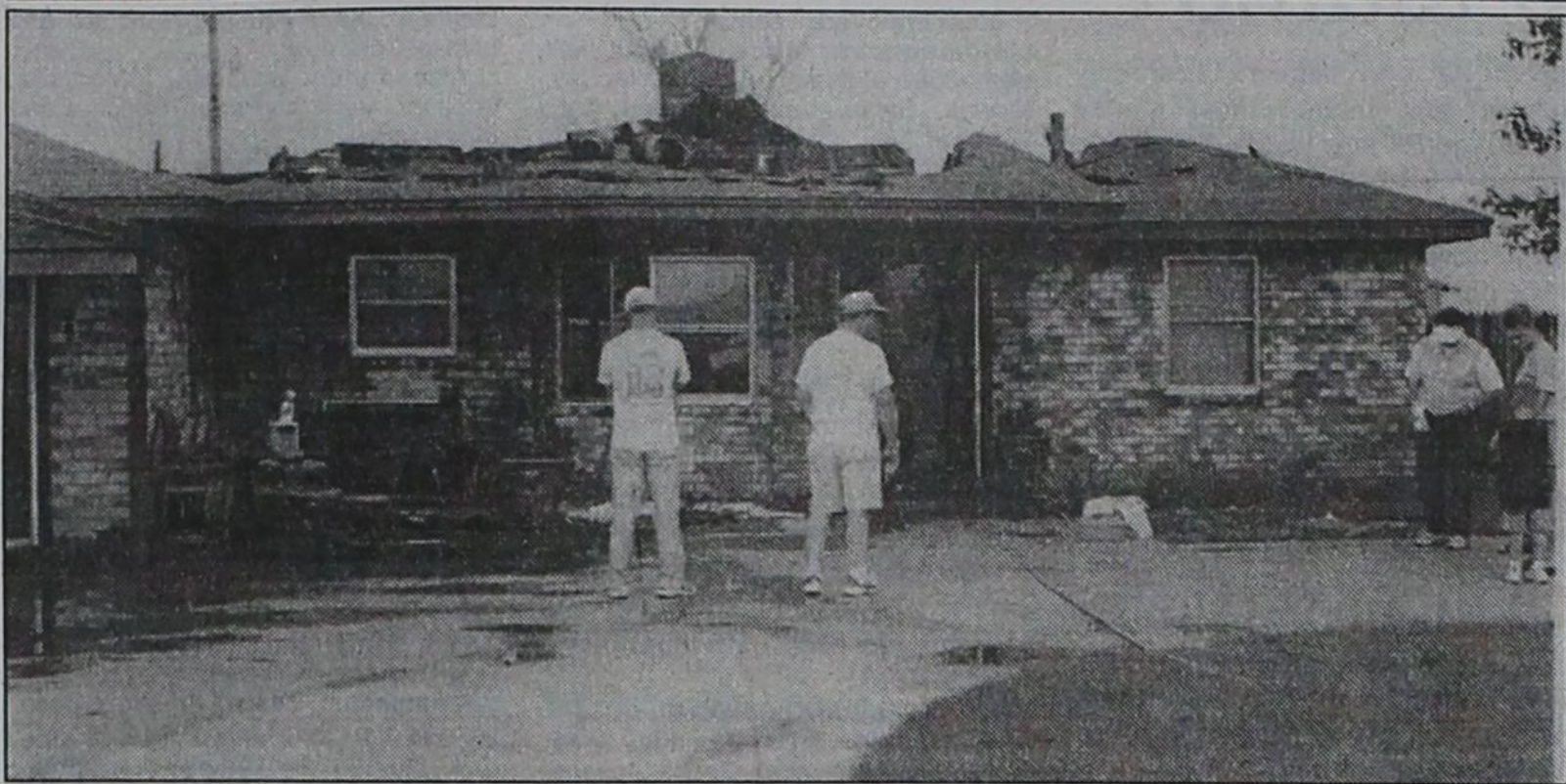
NO ROOF —Early Saturday morning, flames spread through the attic of the Dub George home in Dimmitt on South US 385, consuming a good portion of the roof and causing extensive damage to the home.
