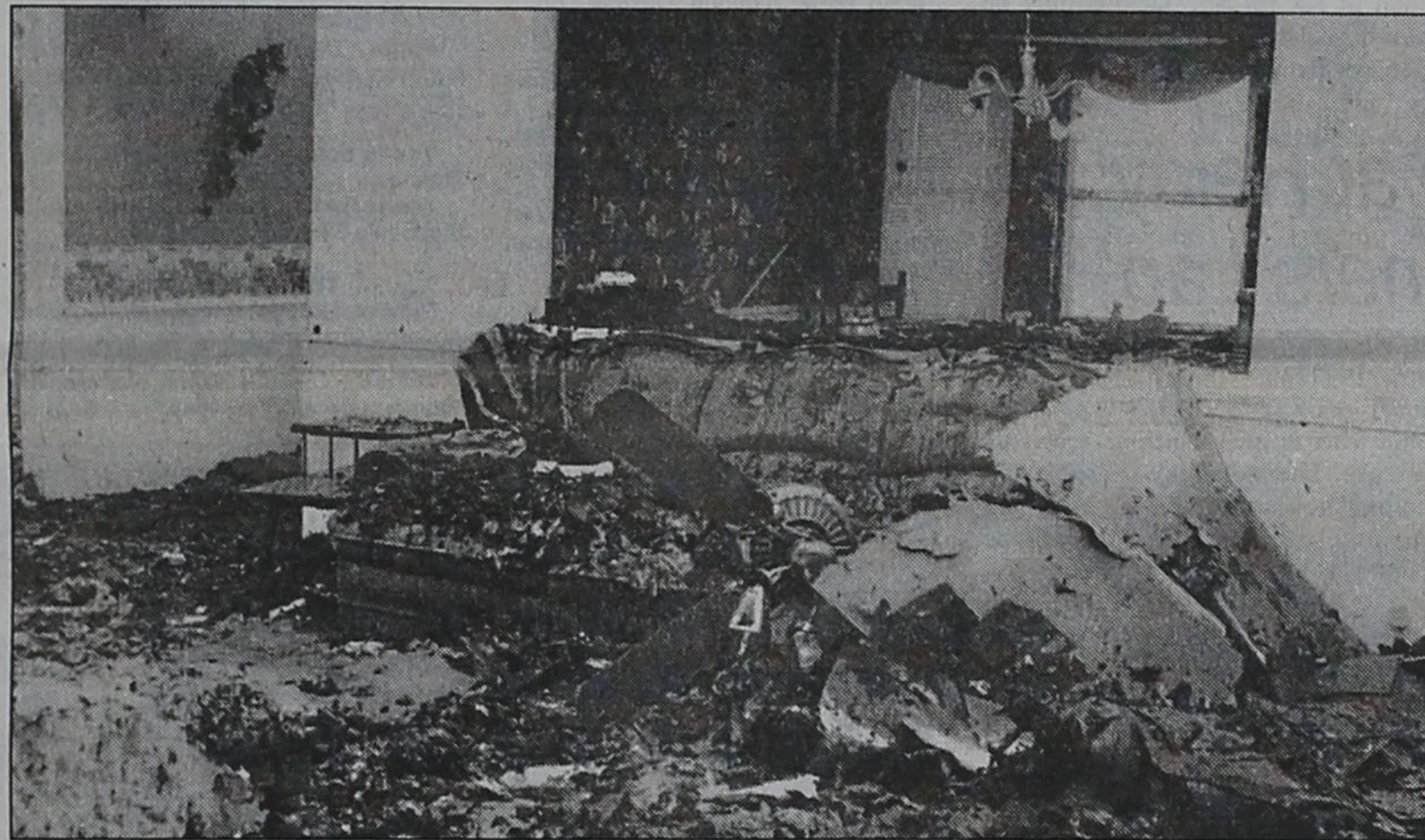
IT'S ALL INSIDE —A lot of what was left of the roof, attic and insulation fell into the house, causing more damage in addition to smoke and water damage.
