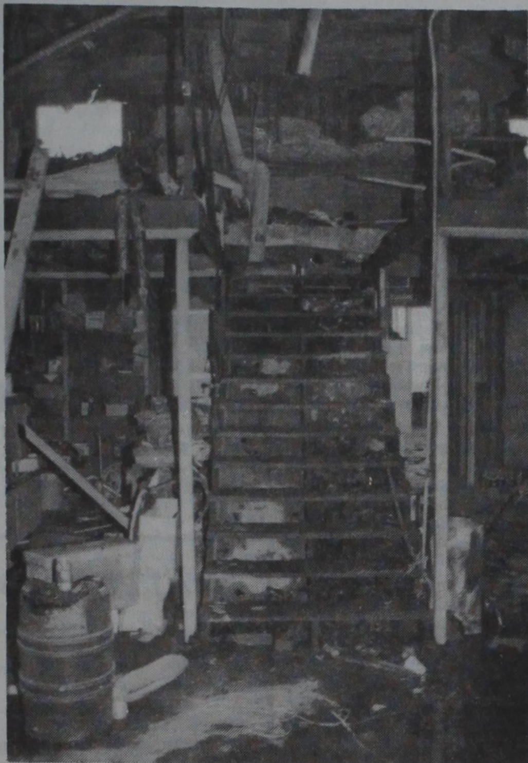
TOASTED STAIRCASE —These stairs lead to the storage loft in the shop area at Dimmitt Ready Mix. The loft and items stored there were totally damaged by a fire Sunday afternoon. The fire started in the shop area, but the exact cause has not been determined yet. No injuries were reported, but the building sustained some structural damage. No dollar estimate has been given yet on the damages.
