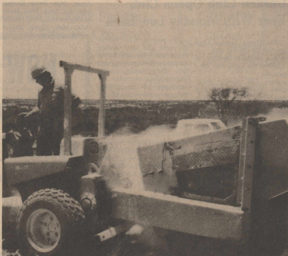
ROCK SAW RIPPER IN OPERATION —General Telephone lineman, Eddie Rogers, operates the ripper on the San Angelo-Ozona project. This is just one of the many units of equipment which are placing more than 600,000 feet of buried cable to provide improved and expanded long distance telephone service to this area. Long distance service, the source of many complaints in Ozona for some time, should be greatly improved when the project is finished.
