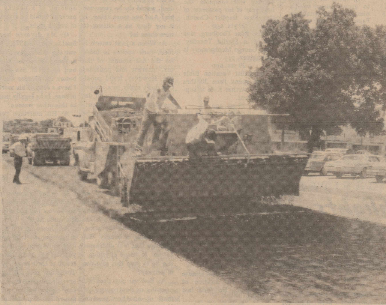
MOST OF THE ACTION this week in downtown Ozona was centered around the paving of State Highway 163 and U.S. Hwy. 290 by the State Highway Department. Traffic lanes were paved separately, causing the minimum amount of
