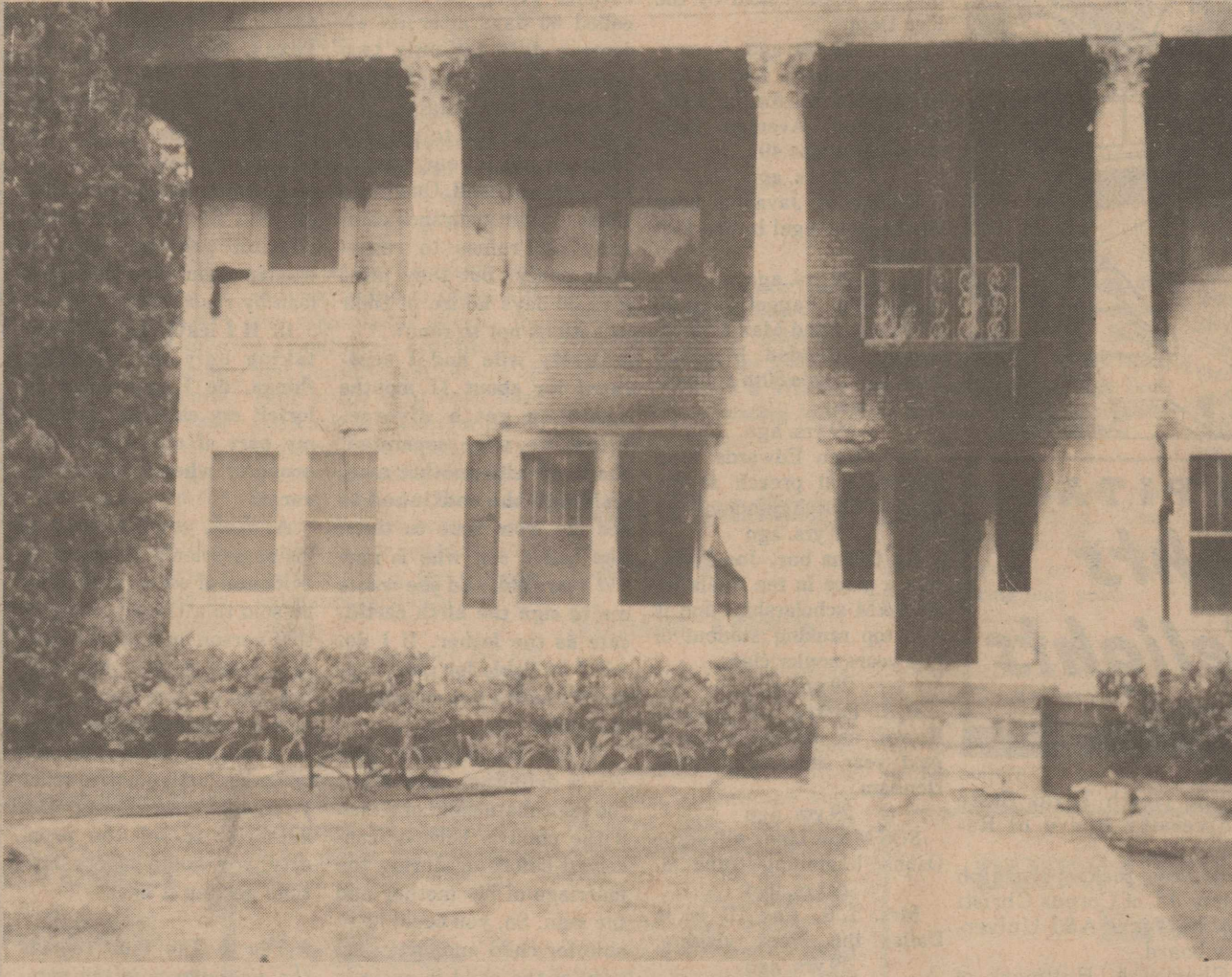
BURNED EXTERIOR OF WAY BACK WHEN -The result of fire which started in the lobby area of the restaurant shortly after midnight, May 18. Eight persons were trapped in the club above the restaurant and barely managed to escape through a bolted door to the fire escape. Fire officials strongly suspect arson and investigation into the blaze continued through press time Tuesday afternoon.
