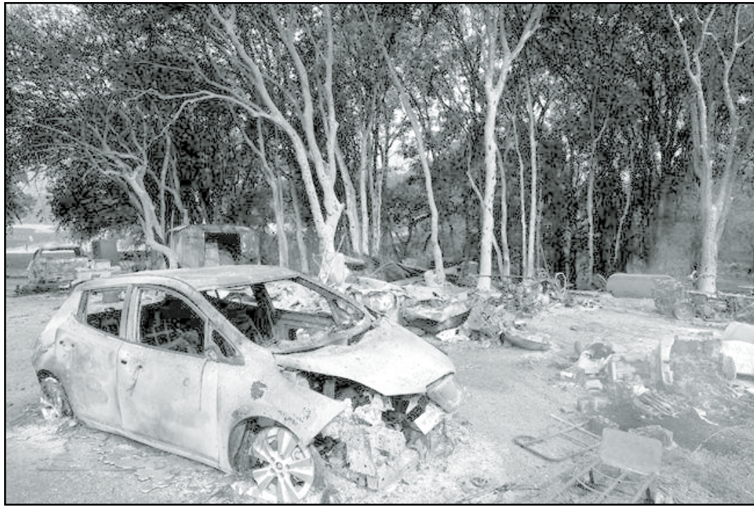
A burned car is seen in front of a wildfire ravaged home Tuesday, July 31, 2018, in Lakeport, Calif. Battalion Chief John Messina said Tuesday fire crews slowed the spread of one of the blazes into towns near Clear Lake, including Lakeport, a city of 5,000. He says the fire instead spread into the Mendocino National Forest.
