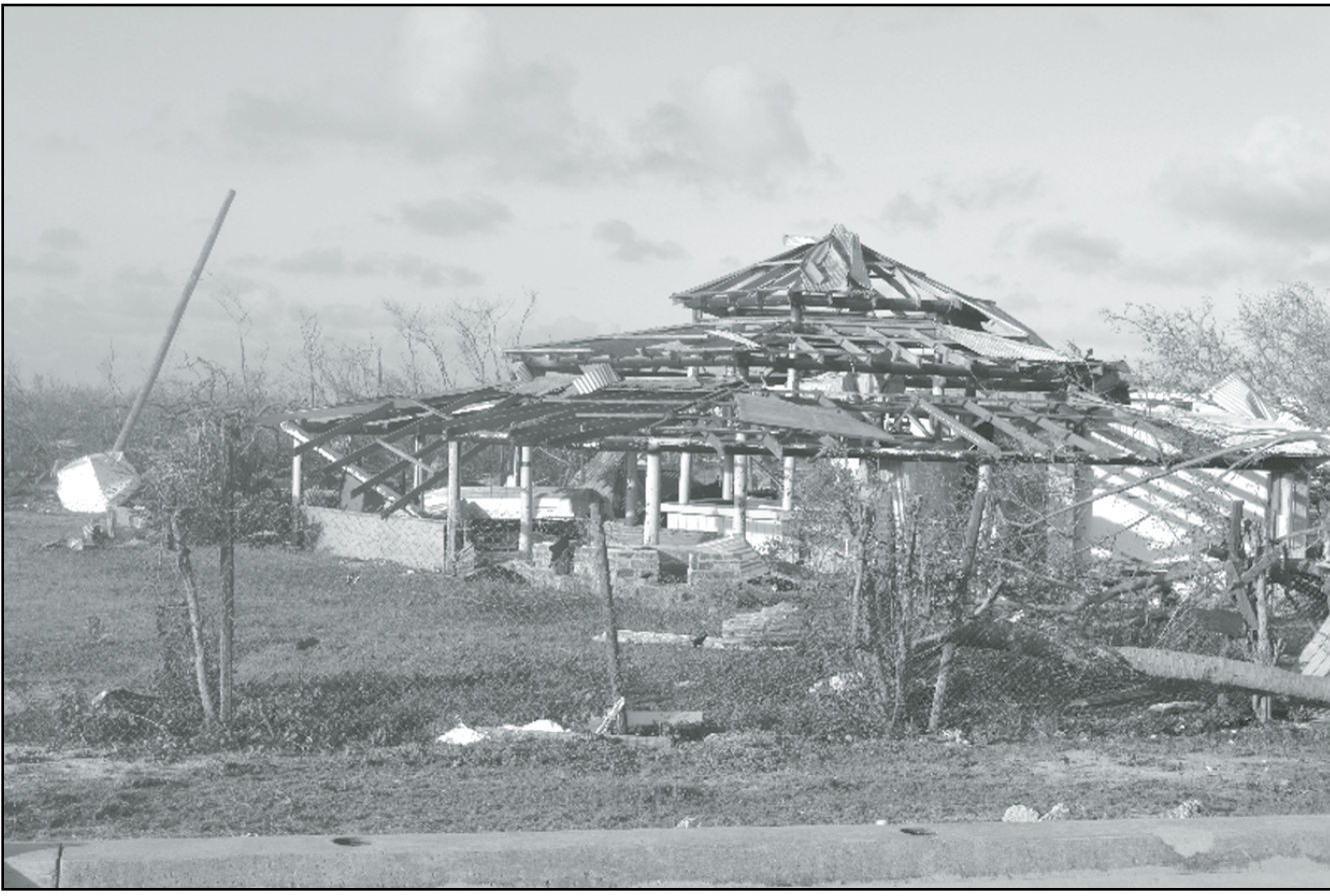
In this Thursday, Sept. 7, 2017, photo, damage is left after Hurricane Irma hit Barbuda. Hurricane Irma battered the Turks and Caicos Islands early Friday as the fearsome Category 5 storm continued a rampage through the Caribbean that has killed a number of people, with Florida in its sights.
