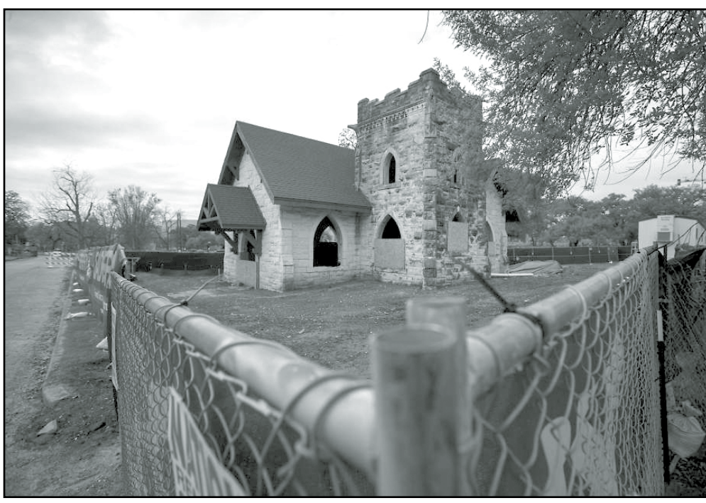
Ralph Barrera/Austin American-Statesman via AP In a March 7, 2017 photo, rehabilitation work of the Oakwood Cemetery chapel, in the heart of downtown area of Austin, Texas, has come to a halt after construction crews discovered human remains underneath it. The chapel is fenced off but access to the cemetery remains open.
