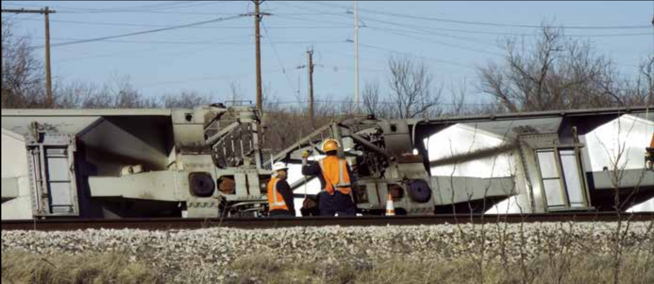
Union Pacific crews clean up and repair track after a minor trail derailment occurred in Big Spring Sunday.
