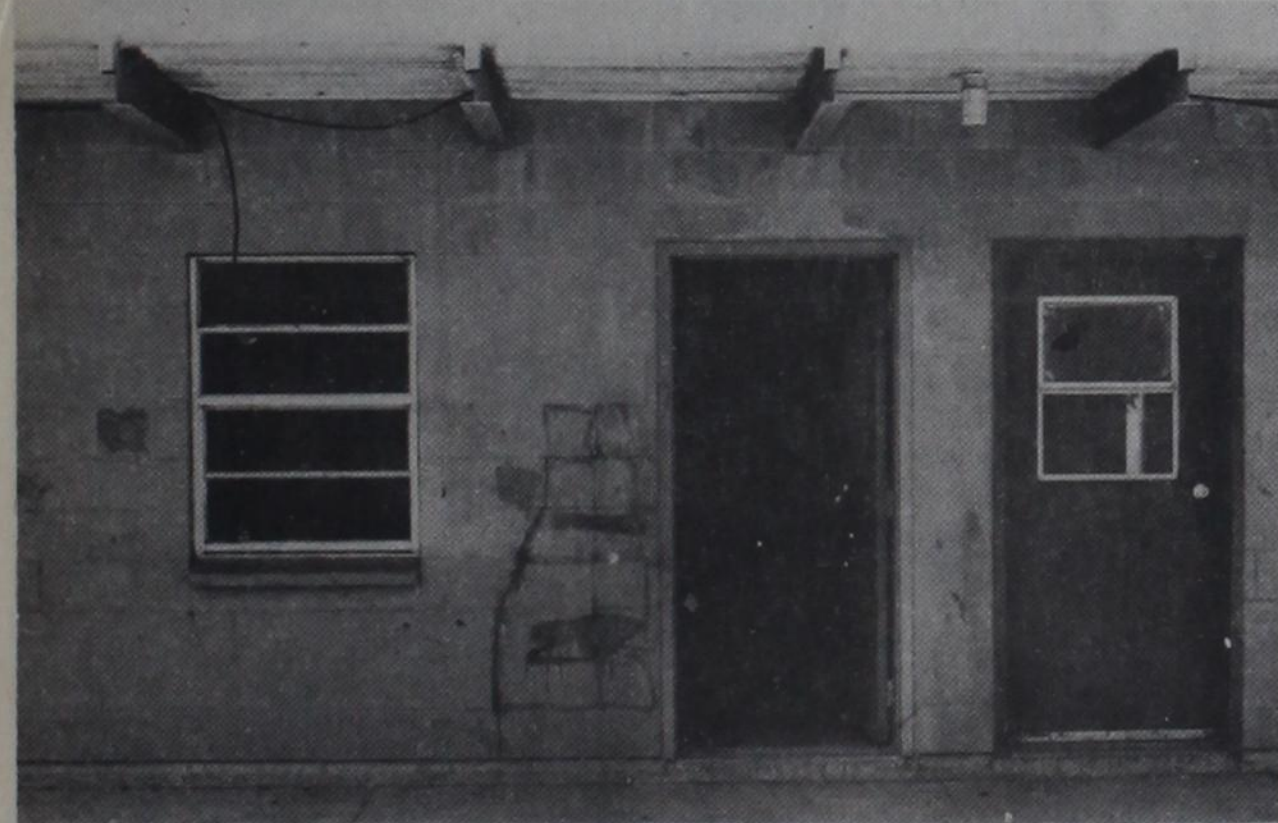
STANDING VACANT—While many permanent workers' apartments at the Castro County Agricultural Housing Project are well-kept, many "seasonal" apartments—such as these—stand vacant as the result of vandalism and lack of maintenance. Due to a
