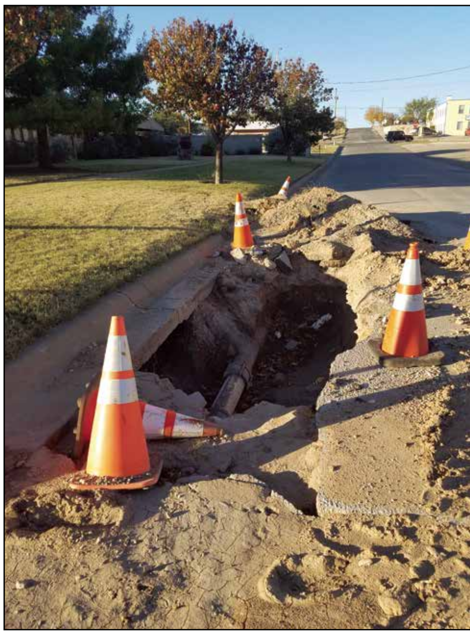
This hole located on 8th St. is one of many across the city that has been open for months. City officials say a rash of broken water lines plus a wet November and limited staff contributes to the delay to fix the holes.
