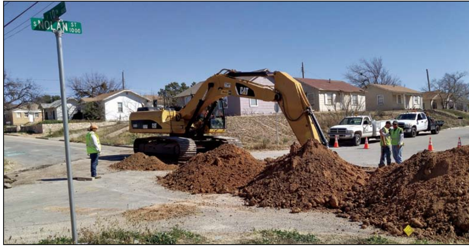
A two-block stretch of Tenth Street from Goliad to Johnson has been blocked off to allow city crews to replace a 20-inch water line. The work began Wednesday and is expected to be completed within the next few days.
