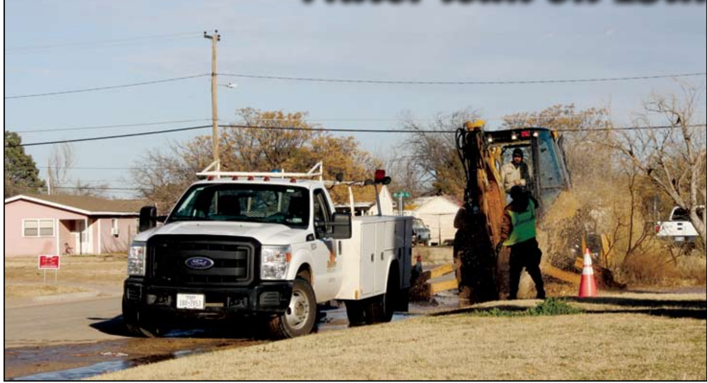
City of Big Spring Utilities workers worked a water leak on East 15 th Street near State Street Thursday afternoon.
