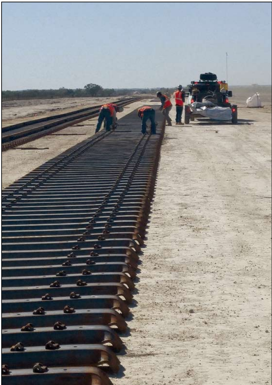
HERALD photo/Steve Reagan Crews work on a railroad switch line that will be part of the Permian Rail Park, a $10 million project under construction west of Big Spring. The facility, which will be used to transport oil fracking material to job sites, is expected to be operational by early 2016.
