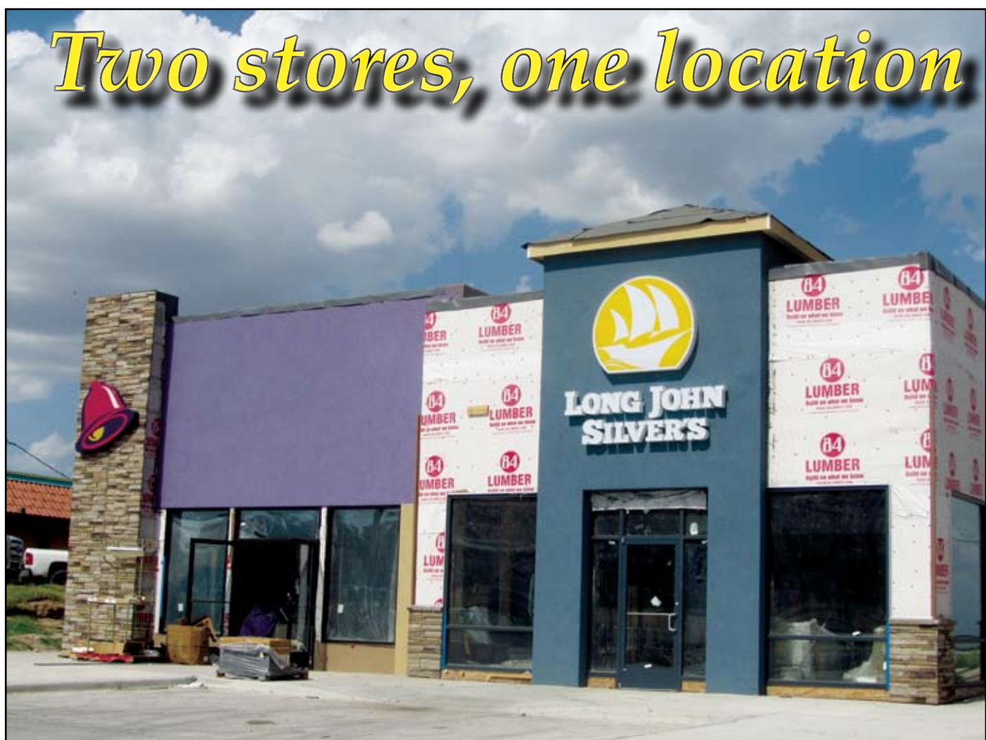
Big Spring will soon have two new fast-food establishments, both at one location. Construction on the building housing the joint Taco Bell/Long John Silver's operation on South Gregg Street is nearing its final stages.
