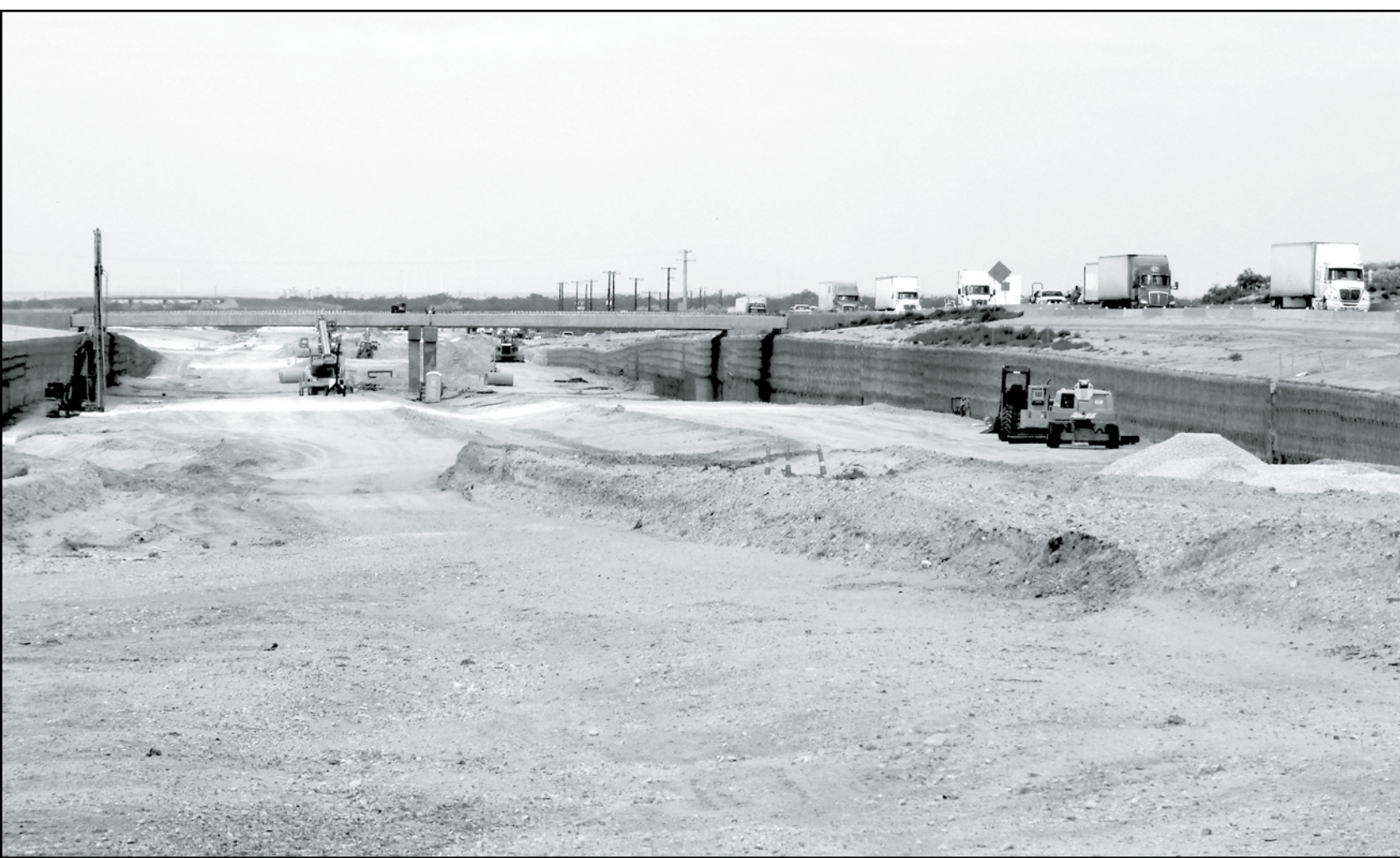
HERALD photo/ Lyndel Moody Work continues on the Highway 87 reliever route immediately west of Big Spring. When this leg of the construction project is completed, it will stretch from Interstate 20 to Highway 87 south of town.
