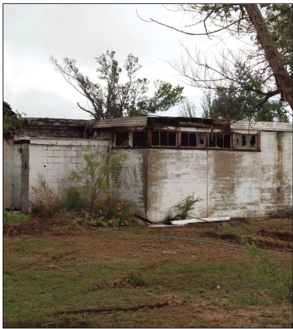
HERALD photo/Steve Reagan Fire destroyed the old Midway School building on Midway Road Monday morning.
