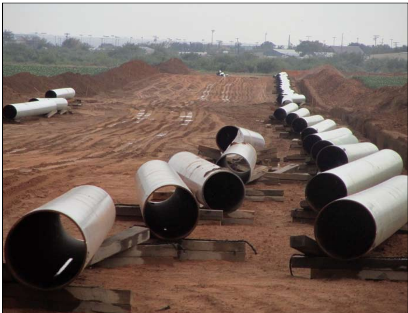
A large crude oil pipe line project by Plains All America is running through Howard County. The Sun Rise pipe line, which is being constructed by Two Rivers Pipeline & Construction, will extend to Colorado City.
