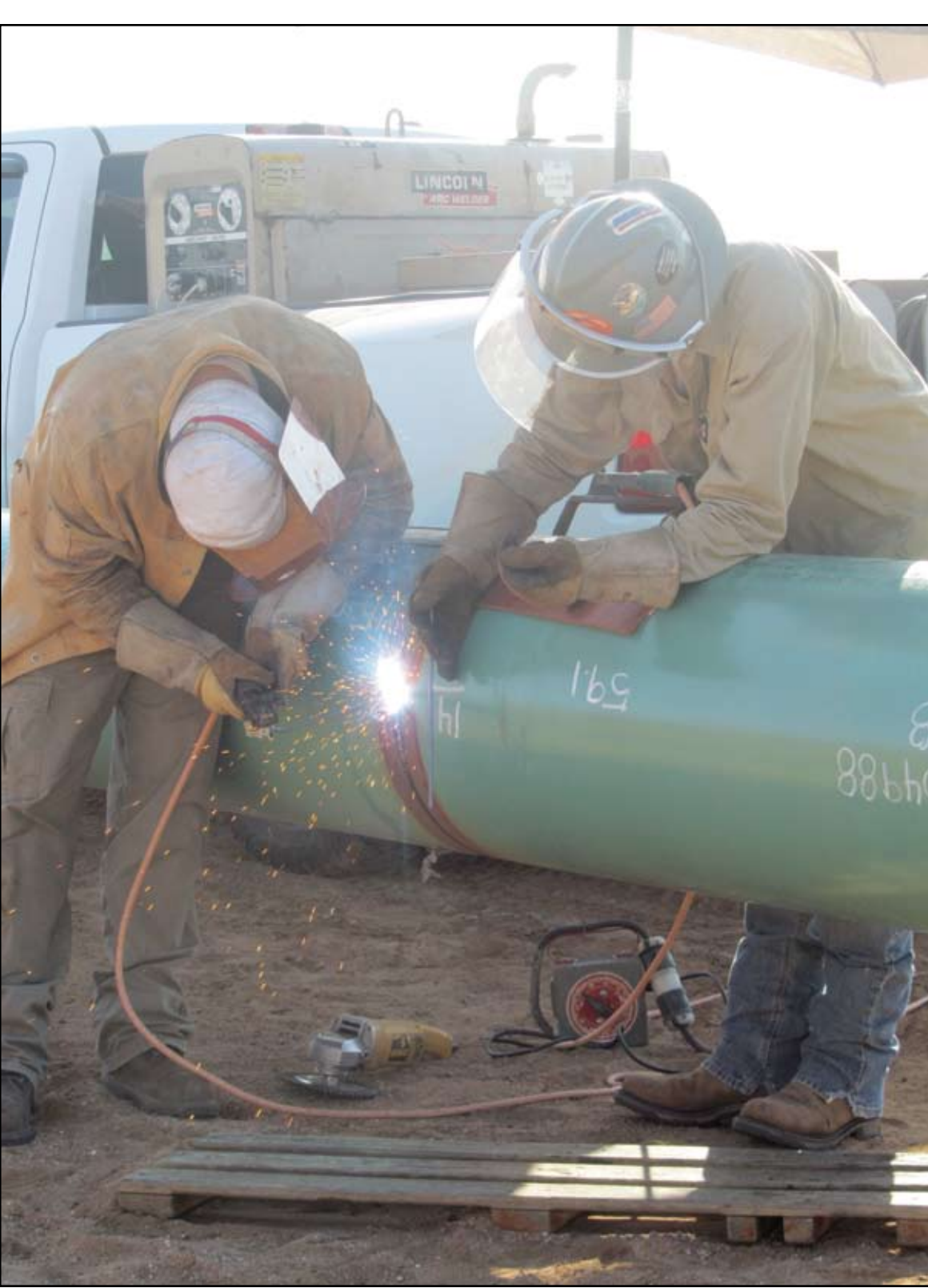
HERALD photo/Lyndel Moody Employees weld 20-inch pipes together this morning as part of a large crude oil pipe line project by Plains All America. The Sun Rise pipe line, which is being constructed by Two Rivers Pipeline & Construction, will extend to Colorado City.
