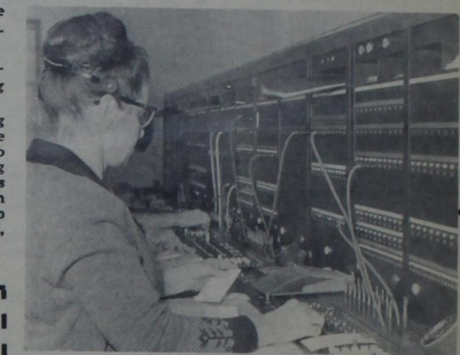
VELMA HOLLAND assists subscribers in completion of long distance telephone calls at switchboard in central office. The new facility provides for five operators. —Staff Photo
