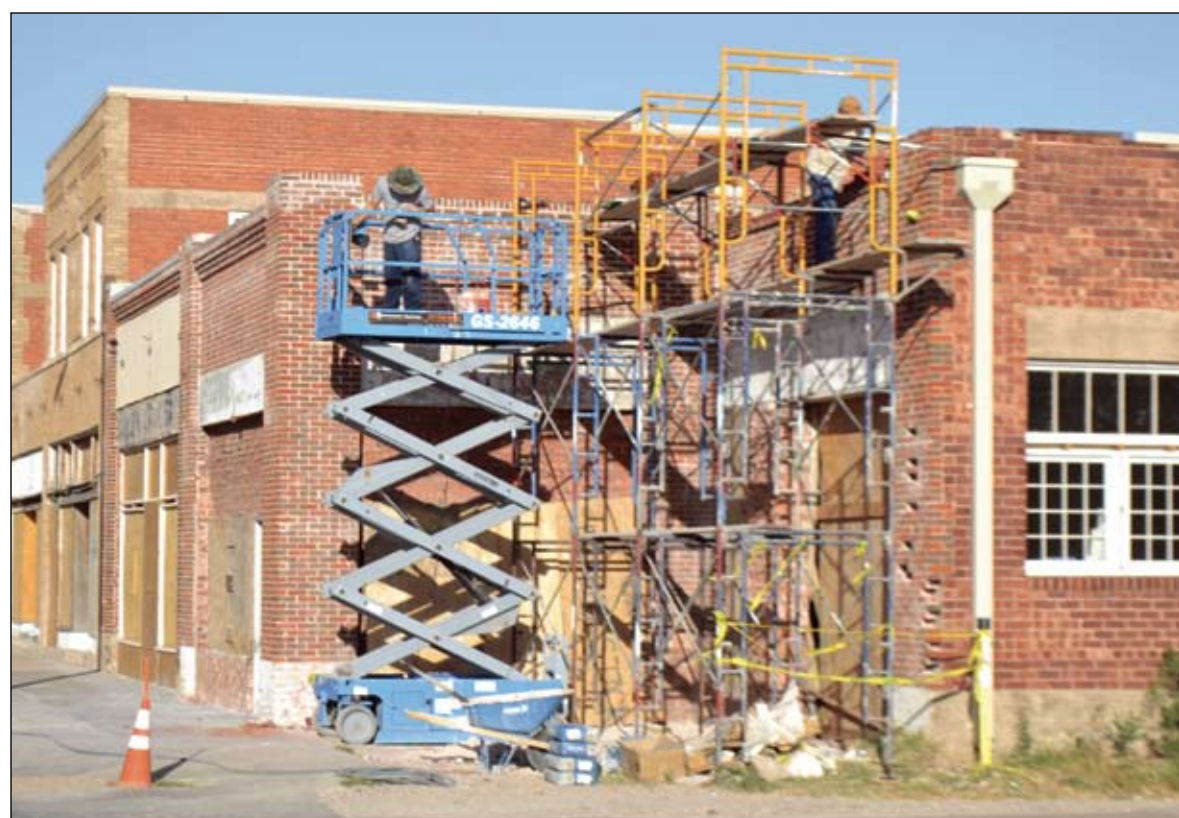
HERALD photo/Steve Reagan Atop a maze of scaffolding, workers were repairing masonry on this building across from the Hotel Settles on East Third Street today.
