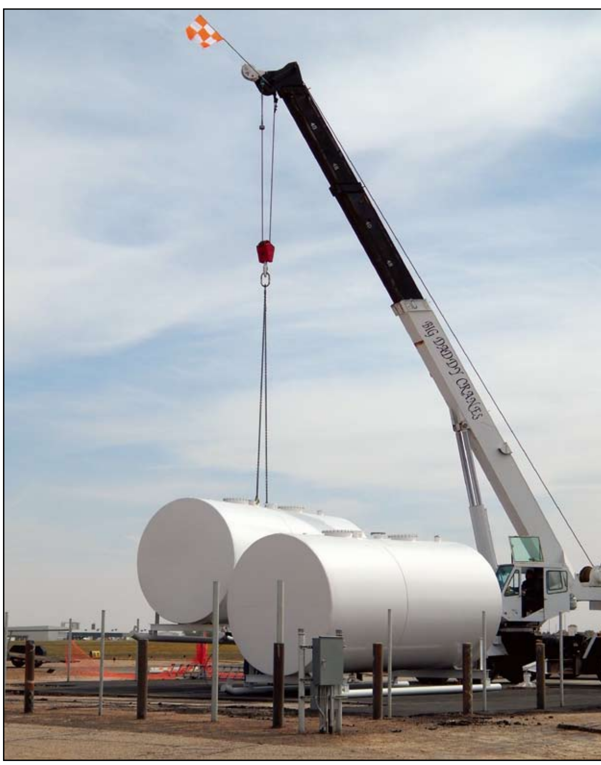
Work crews place two 12,000-gallon tanks just west of the main runway at Big Spring Airport Wednesday morning. When installation is complete, the new tanks will give pilots a self-serve option when refueling.
