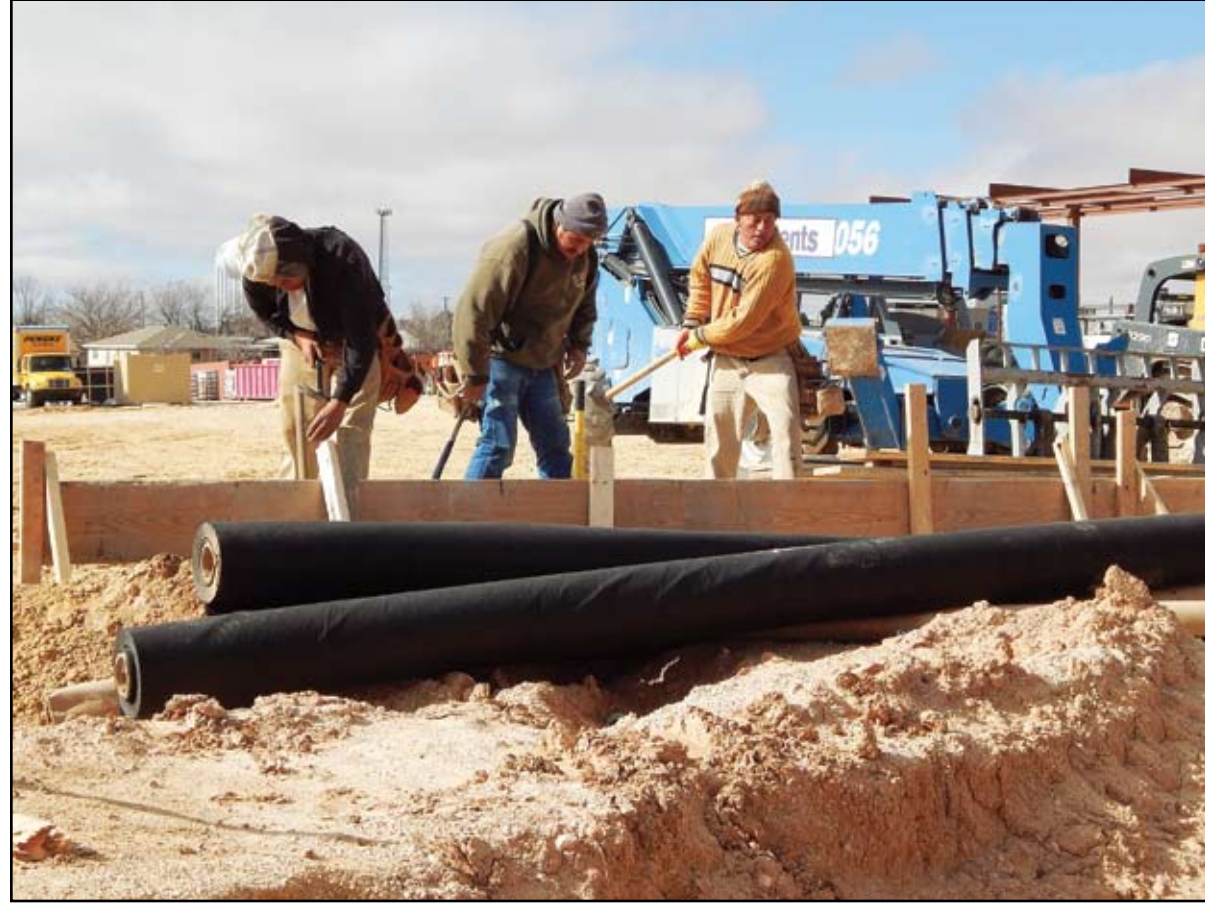
HERALD photos/Andrea Medlin Construction continues at the site of the Pilot Travel Center. In the bottom photo, from left, Juan Barreto, Hugo Gomez and Juan Vilcheg drive wooden planks into the ground near the fuel pumps. The center is set to open early next year and is located on the south service road at the intersection of Highway 350 and Interstate Highway 20.
