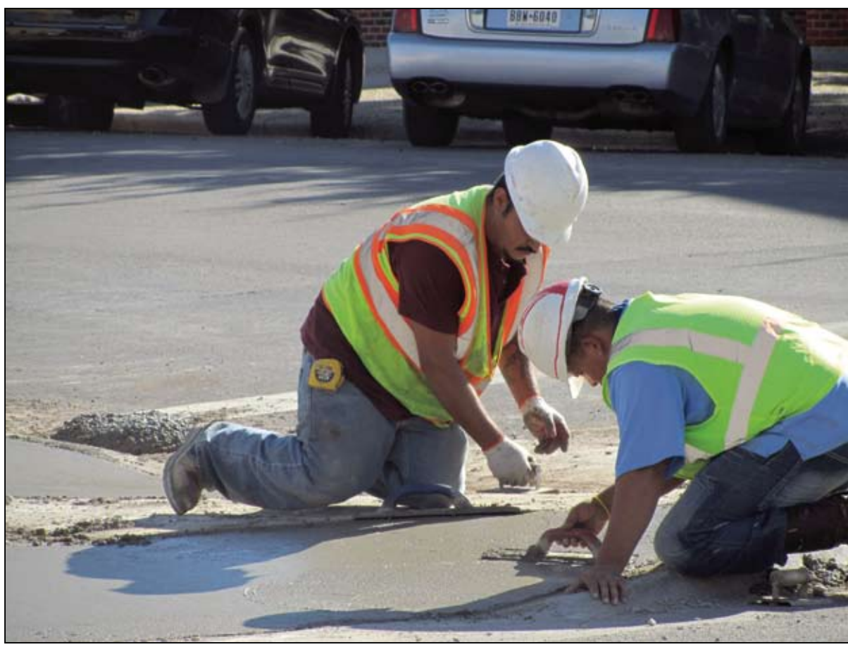
Construction workers smooth out poured concrete on the corner of Fourth Street and Scurry Tuesday afternoon.
