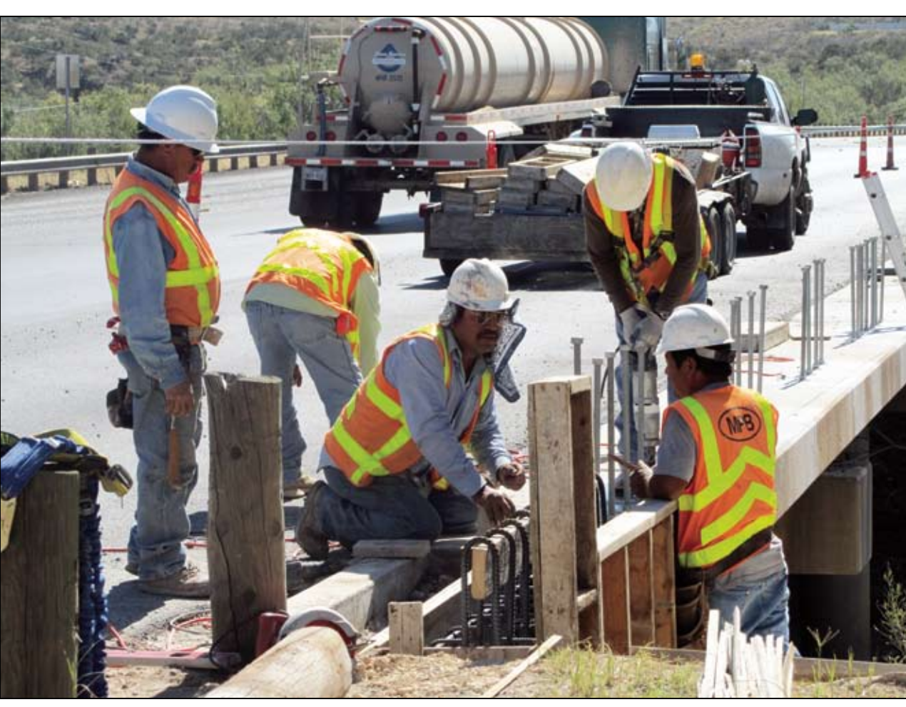
A construction crew from MPB out of Center Point, Texas, works on the guard rail at the U.S. Highway 87 bridge near the Comanche Trail Lake dam Thursday afternoon. South-bound traffic on Highway 87 has been reduced to one lane over the bridge.
