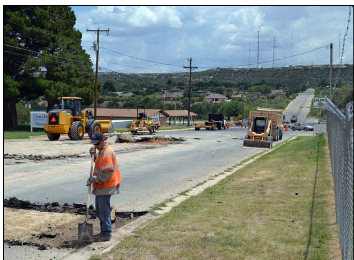
Crews work to repair a stretch of Goliad between 23 rd Street and 24 th Street following the replacement of a water line in the area. Traffic is being detoured west onto 23 rd Street while work is under way. Repairs are expected to be completed and the roadway opened again by Wednesday morning, according to municipal officials.
