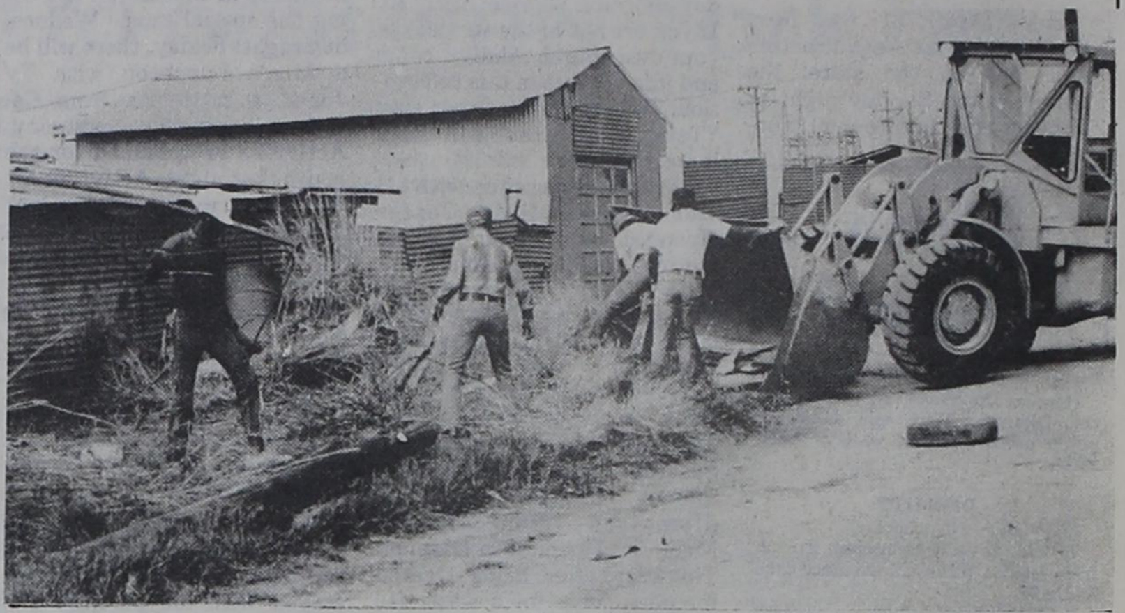
WHEN PUSH COMES TO SHOVE a front end loader helps. Several Dimmitt residents dig their way through litter of all types at the livestock pens between FM 3215 and South
