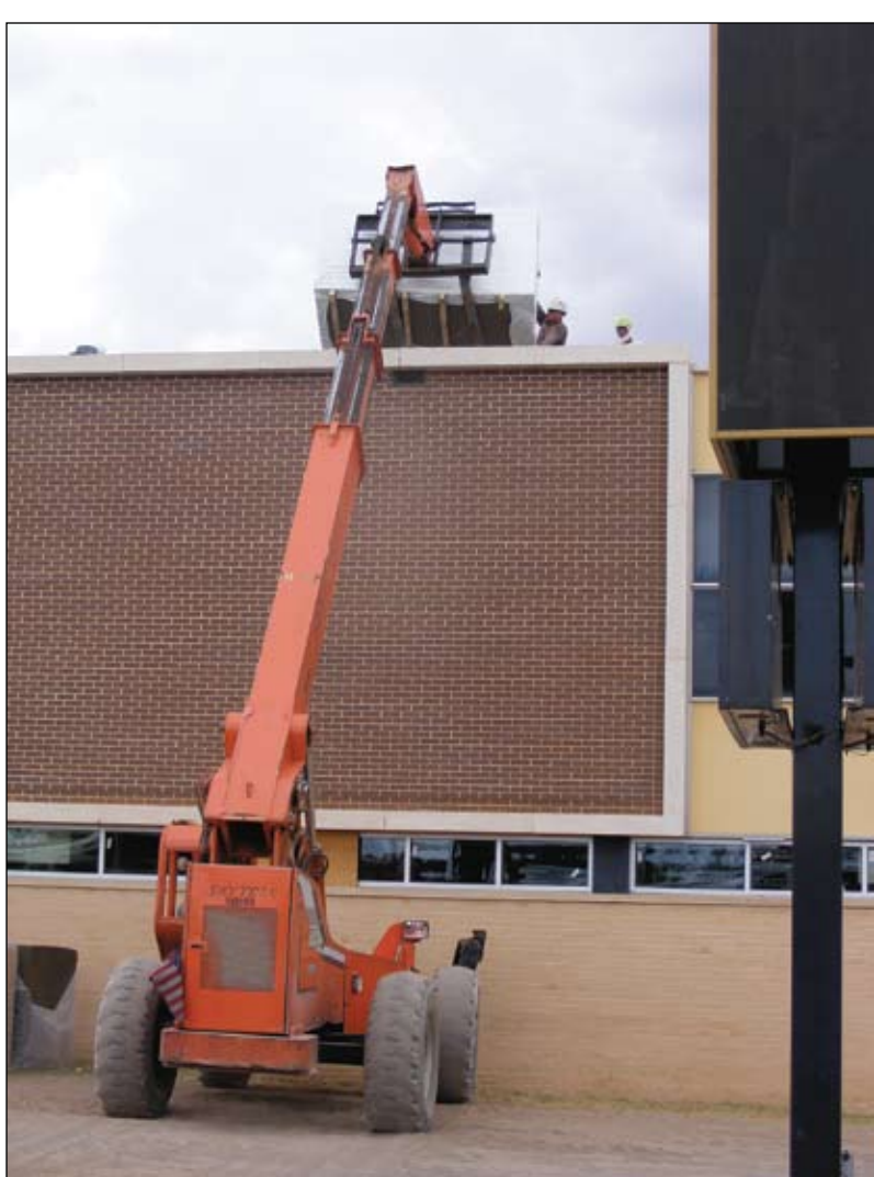
HERALD photo/Steve Reagan Crews raise roofing material to the top of Big Spring High School as renovation work on the building continues. School district officials say work at the campus is expected to continue through February.
