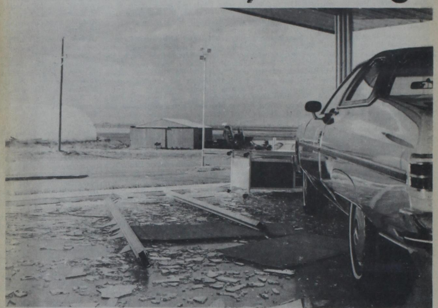
WIND DAMAGE IN SHOWROOM OF REEVE-FLEMING CHEVROLET ... "When the first panel went, the rest went like dominoes"
