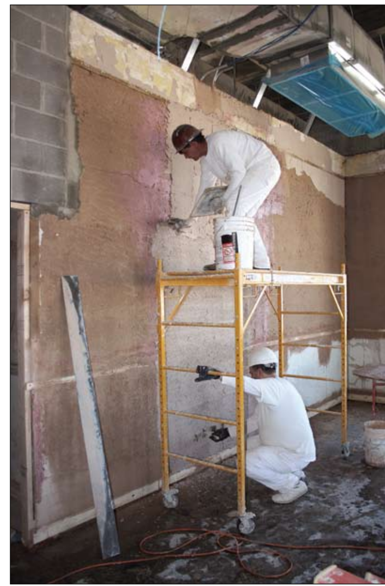
HERALD Photo/Thomas Jenkins These contractors work to repair a wall on the ground floor of the historic Settles Hotel Tuesday afternoon. The hotel — which is currently undergoing restoration — is expected to be reopened to the public later this year.
