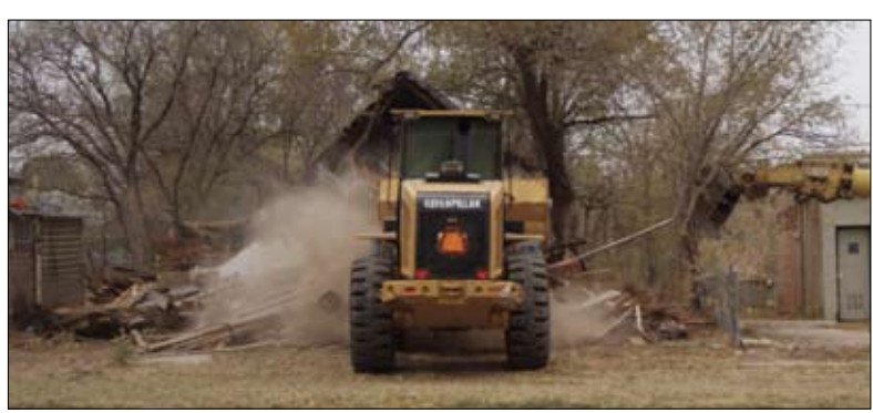
City crews demolish Mary Witkowski's previous residence, which was beyond repair, in order to make room for a new house which will be built by volunteers through the Spring of Siloam.
