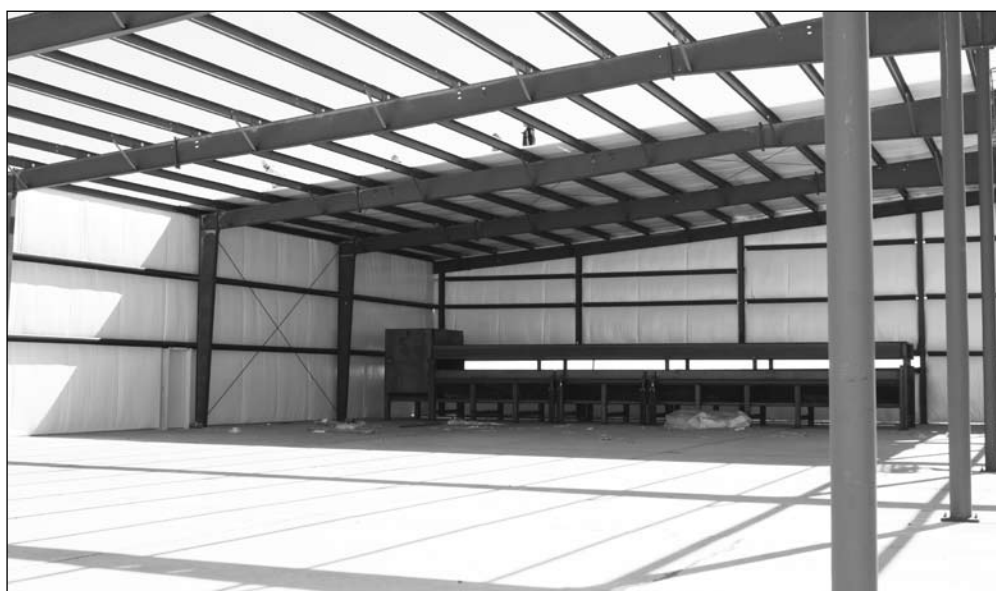
HERALD photos/Amanda Moreno CeRam-Kote, located in the McMahon-Wrinkle Airpark, has recently expanded its facility with the help of Big Spring Economic Development Corporation. The expansion will double the production capacity of the locally owned, family business.
