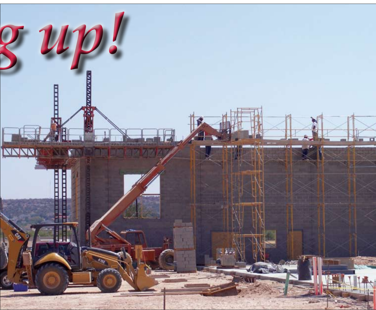
HERALD photo/Steve Reagan Workers erect the walls of what will become the new Goliad Elementary gymnasium Thursday afternoon. The work is part of a $60 million construction project that will result in four new elementary buildings and renovations to other Big Spring Independent School District campuses.
