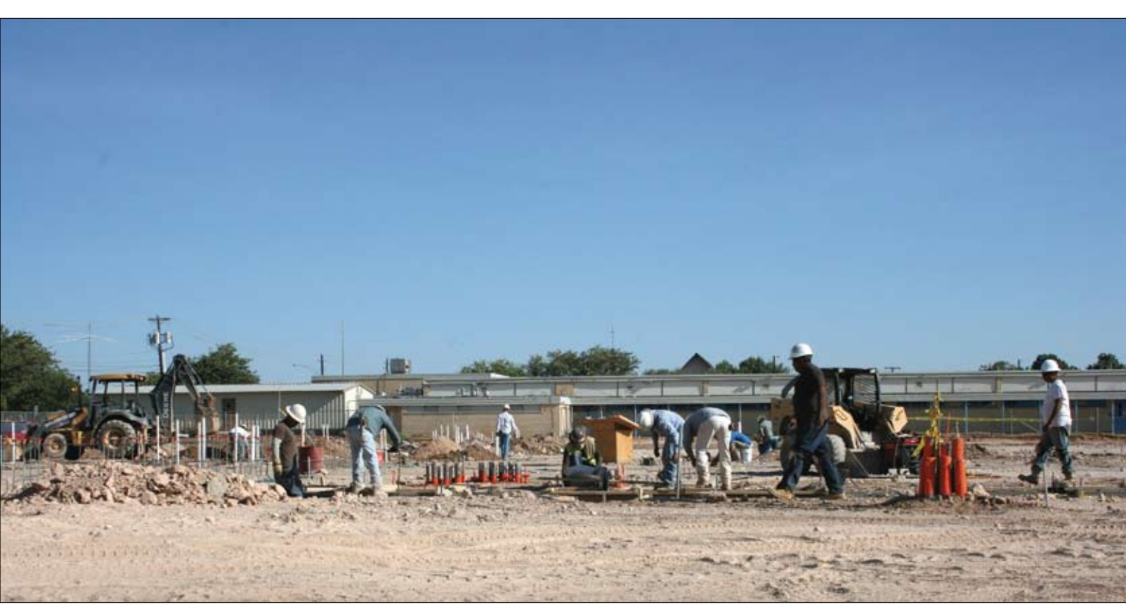
Work continues on the site of what will soon be the new Washington Elementary campus — located adjacent to the old campus on Birdwell Lane — as the Big Spring Independent School District continues its multi-million dollar project to replace several aging schools throughout the city.
