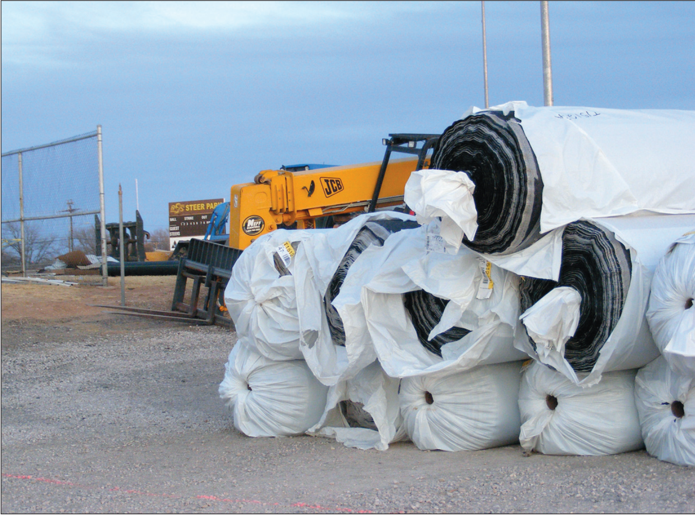
Bundles of artificial turf material are stacked adjacent to Steer Park Sunday evening. Installation of the new baseball surface should be completed by Jan. 15, officials said.
