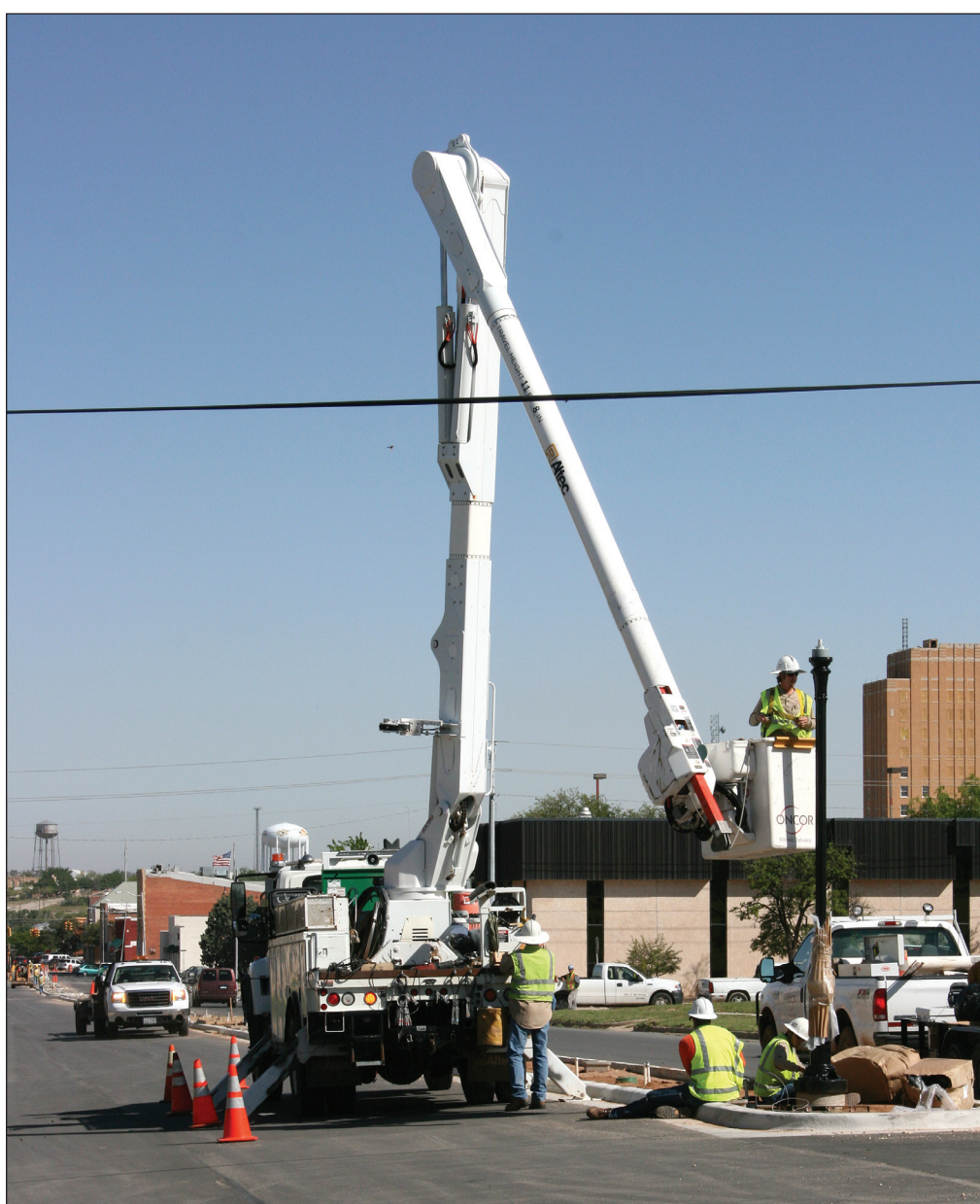
HERALD Photo/Thomas Jenkins Contractors with Oncor Electric work to erect a street light in one of the medians located on Main Street. The lighting is part of the city's downtown street project, which calls for streetscaping in and around the downtown area.
