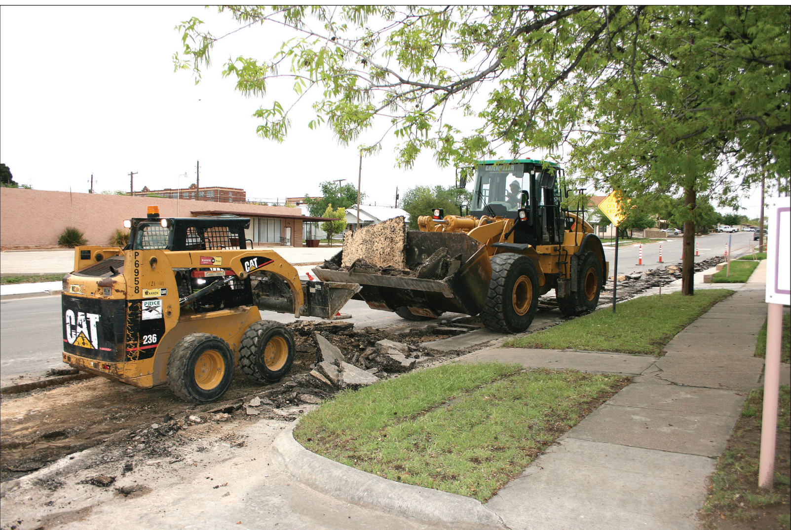
HERALD Photo/Thomas Jenkins Workers with Price Construction tear up a stretch of newly resurfaced Scurry Street in the 800 block Monday. According to city officials, the construction company is having to replace the surface because of cracking and moisture problems. The roadway was recently resurfaced as part of the city's bond-funded street renovations project aimed at downtown Big Spring, with this most recent replacement coming at no charge to the city.
