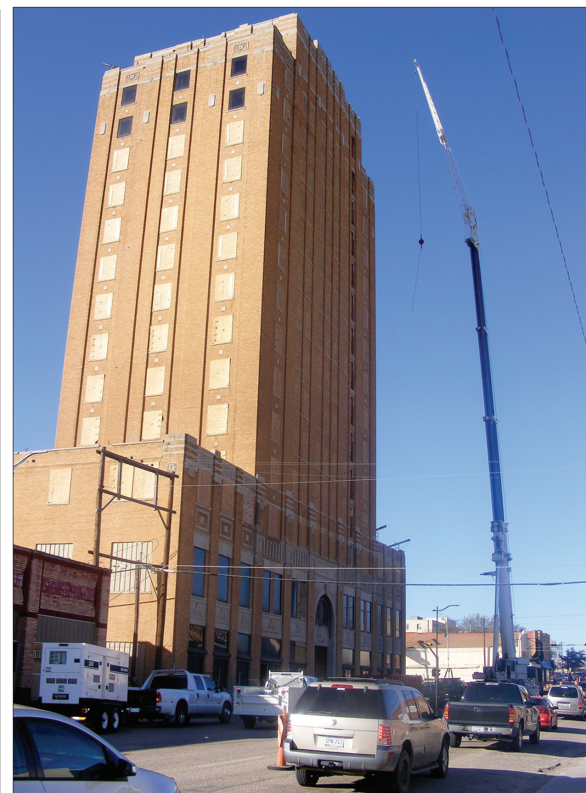
HERALD photo/Steve Reagan Work crews set up a crane outside the Settles Hotel building this morning. The crane will be used to hoist elevators to the top of the building.
