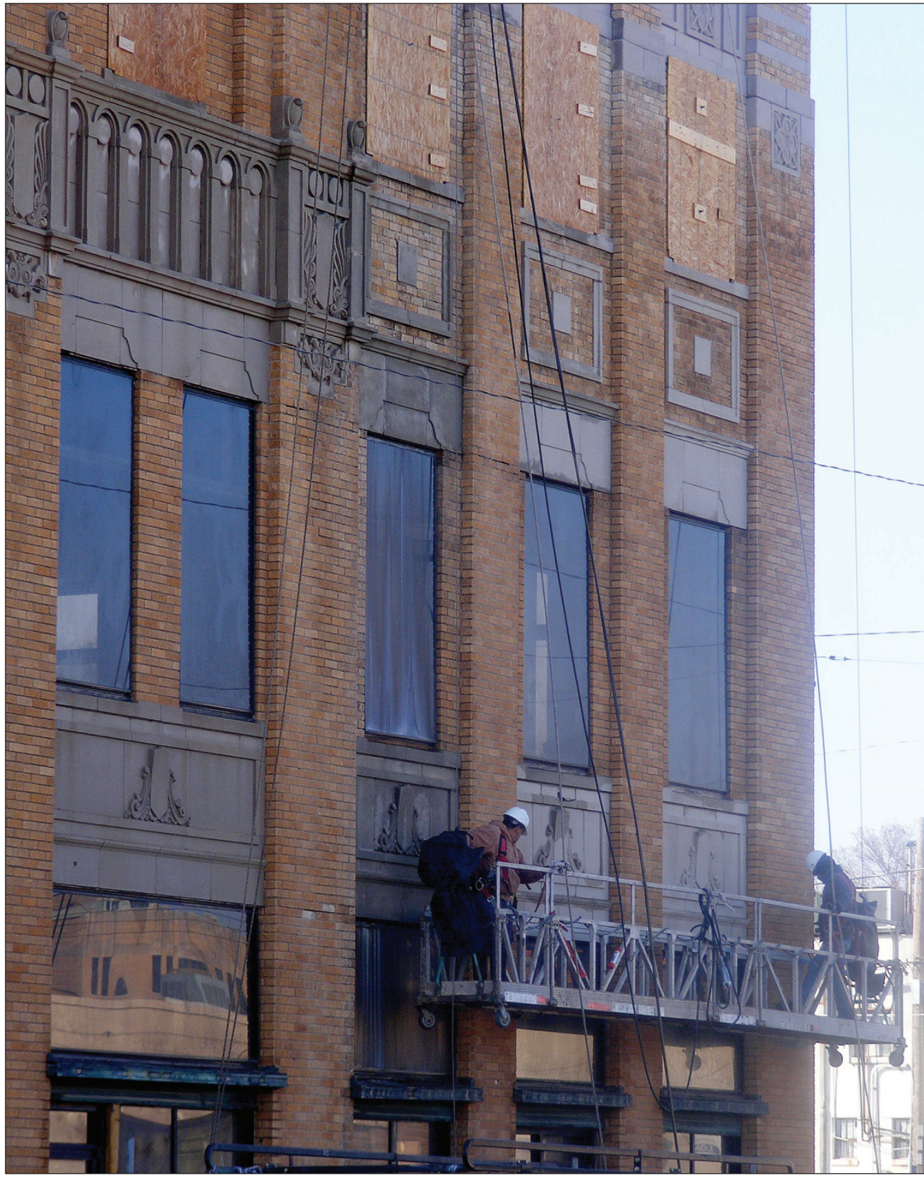
Crews from D&S Construction use a scaffold as they perform renovation work on the exterior of the Settles Hotel Friday morning.
