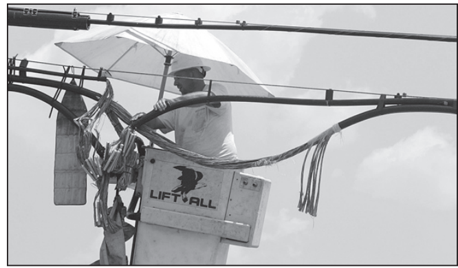
AP Photo/The Courier, Eric S. Swist A telecommunications line worker keeps cool under a large yellow umbrella as he services damaged phone lines in Conroe Friday.
