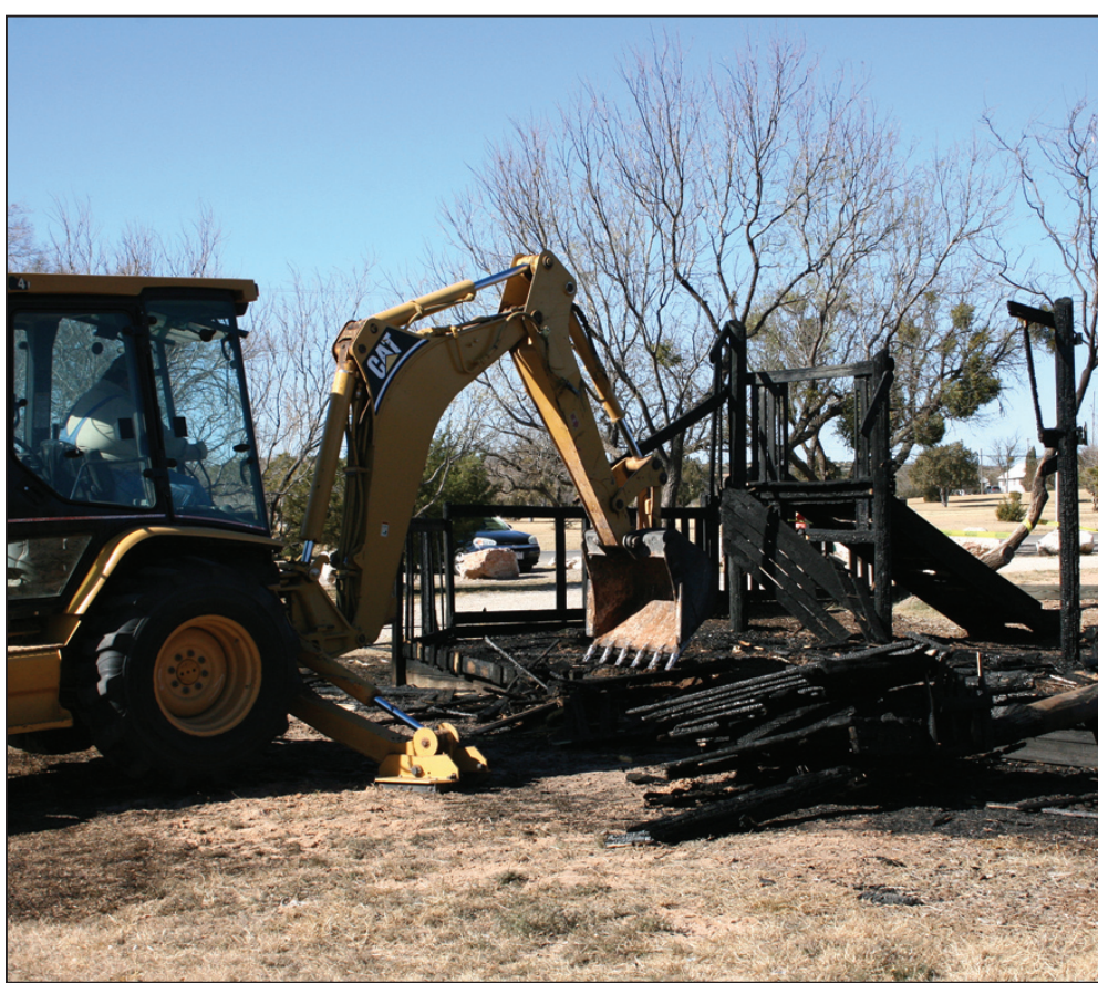
HERALD Photo/Thomas Jenkins A city employee uses this back-hoe to clear away the remains of a portion of Kids Zone in Comanche Trail Park after a fire ripped through the facility late Tuesday night. According to investigators, arson is suspected.
