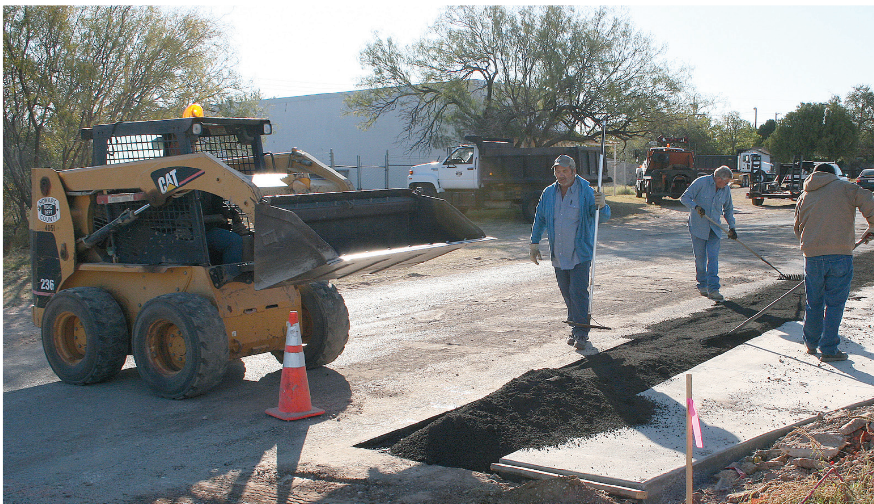
Construction crews work on the entrance area of the new Howard County Jail early Friday morning. Work on the $11.57 million facility is more than 30 percent done, according to county officials, and is on track for completion sometime in March.
